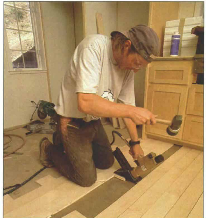
Nailing into the subfloor. Once the subfloor has 6% to 8% moisture content, 4-in. T&G maple flooring is blind-nailed with \frac{1}{2} -in. staples that don't penetrate the slab. Maple is light-colored and moves a lot, so it will show more seasonal gaps between boards than other species.
