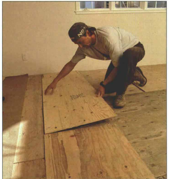
Setting the second layer. The second layer of ½-in. plywood is placed in construction adhesive with joints staggered over the bottom layer. To allow for expansion, ¼-in. wide gaps are left between sheets. At left, kraft paper will act as slip sheet between finish flooring and subfloor.
