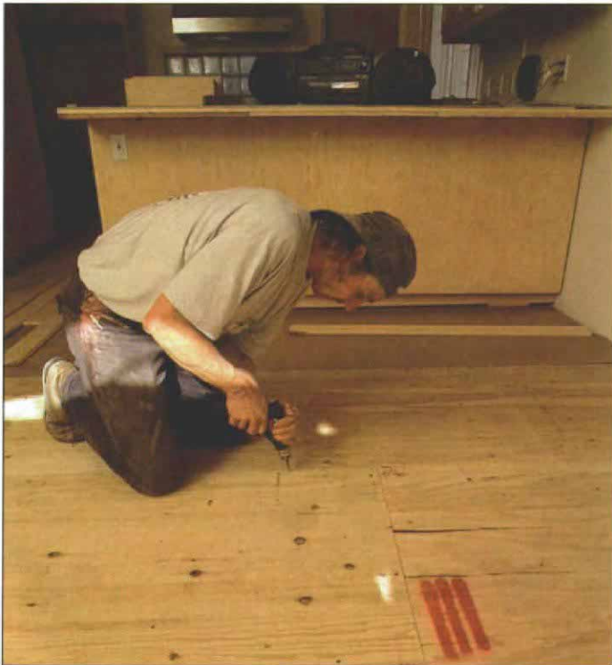
Fastening layers together. The two layers of \frac{3}{4} -in. plywood subfloor are screwed together 1 ft. o. c. with \frac{3}{4} -in. wood screws, which don't go through the bottom layer of plywood. The plywood is screwed together while the adhesive is wet to draw the sheets together.
